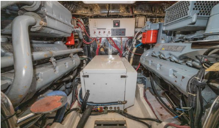
T/CAT 435 HP and ONAN Generator
